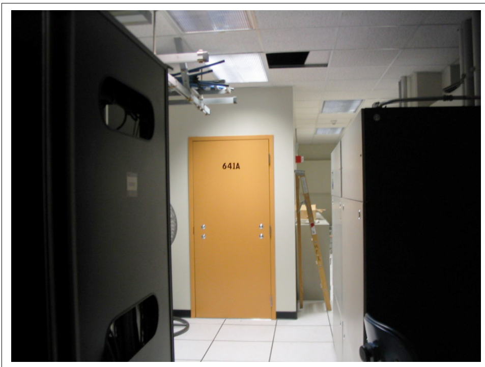
Figure 1-9. Room 641A—NSA interception facility inside an AT&T datacenter in San Francisco
