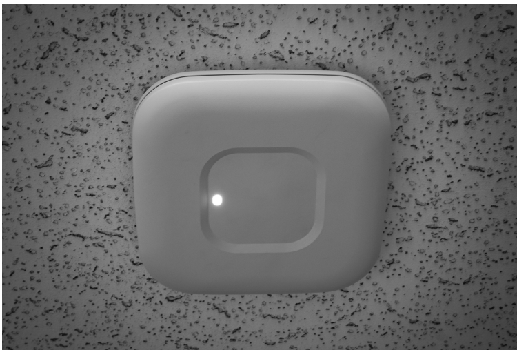
FIGURE 5.9 A ceiling access point Wi-Fi. Courtesy of Shutterstock.
