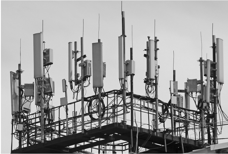
FIGURE 8.9 Multiple Cellular Antennas (3G, 4G, and 5G). Courtesy of Shutterstock.
