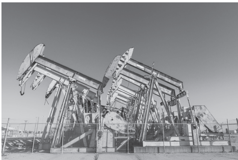
FIGURE 48. Decommissioned pumpjacks on Port of Long Beach land, 2021. Photo by McKenzie Stribich.
